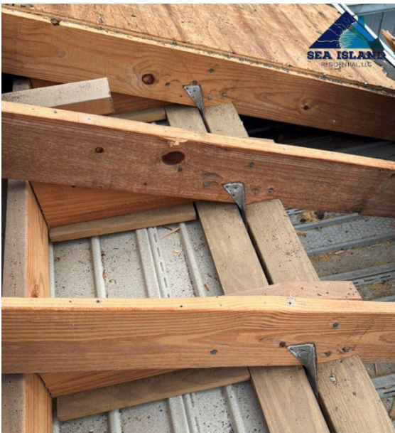
Photo Documentation: Installation of Roof to Wall Connectors (Safe Home Roof Retrofit Requirement)
